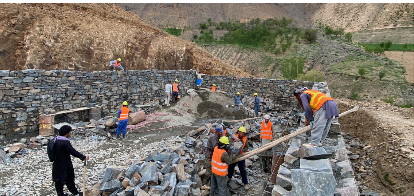
Infrastructure project helped local youth & unemployed community members through providing job opportunities and enhancement of their knowledge and skills in masonry in safe environment.
